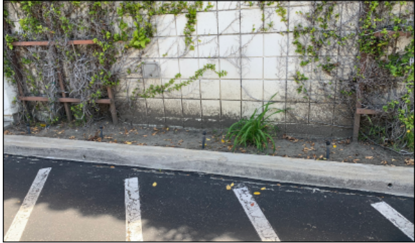
Warehouse Exterior - CMU Water Infiltration
