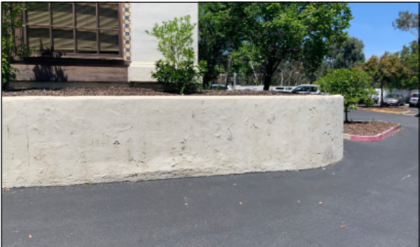
Site Wall - Stucco Condition
