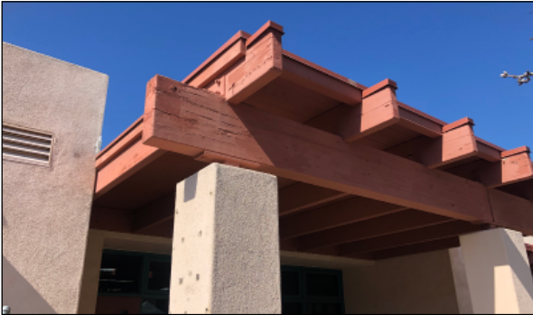
Aging Beams at Kindergarten Building
